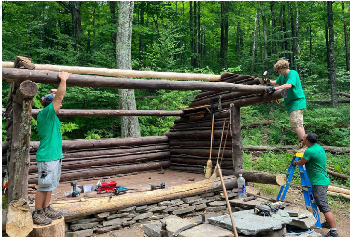
Josh, Liam, and Brandon attaching the front roof beam to the shelter
