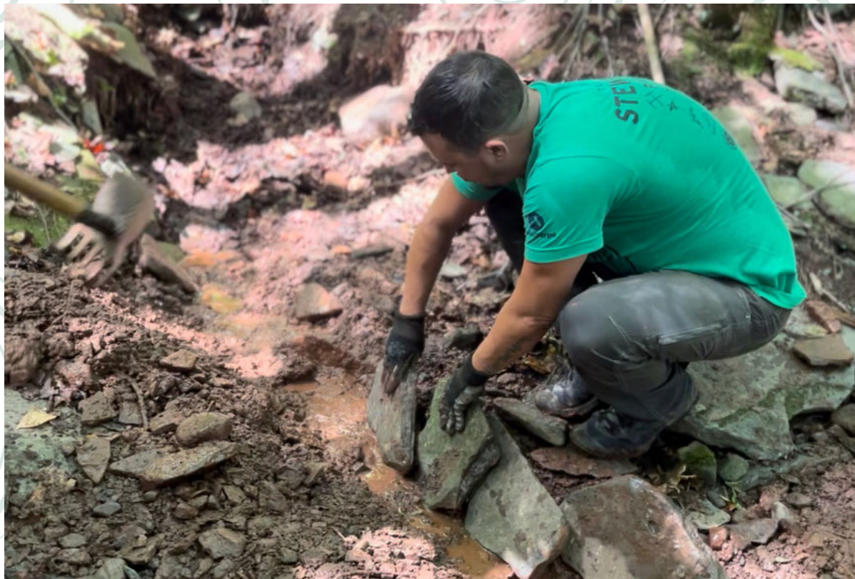
A water bar in the drainage channel will provide structural support and prevent erosion
