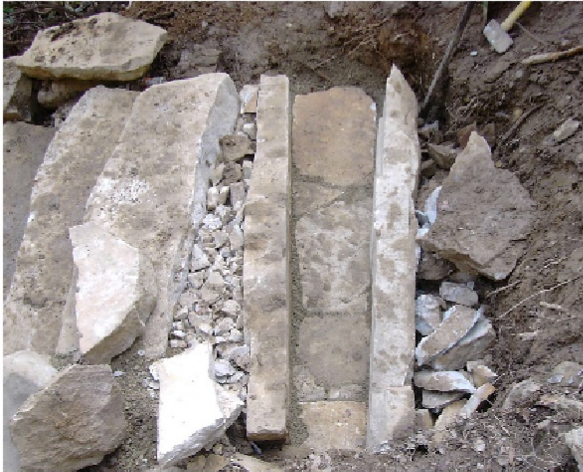
The above stone culvert was installed under a stone staircase - a stone step served as the cap stone on the culvert.
